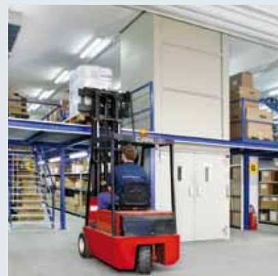
With elevator systems, personnel and goods can easily get to the upper levels
